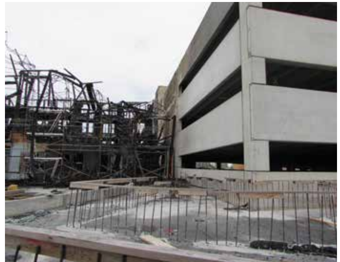
Fig. 2: Another view of the fire damage to wood-framed apartments
