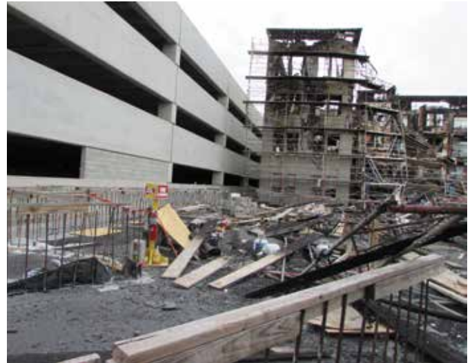
Fig. 1: Fire damage to the apartments at Riverworks at Eastern Wharf
