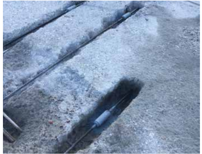
Fig. 8: PT cables had to be spliced with chucks and damaged sheathing repaired
